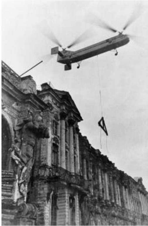
Figure 13. Installation of new trusses over the Great Hall on June 17, 1959. Helicopter commander I.S. Grigoriev
