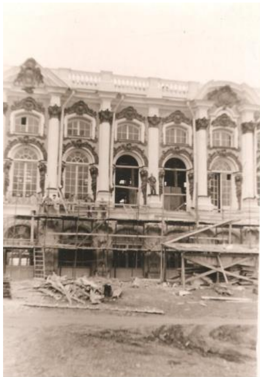
Figure 14. Restoration of the Catherine Palace facades in the Great Hall area. (1960 years)
