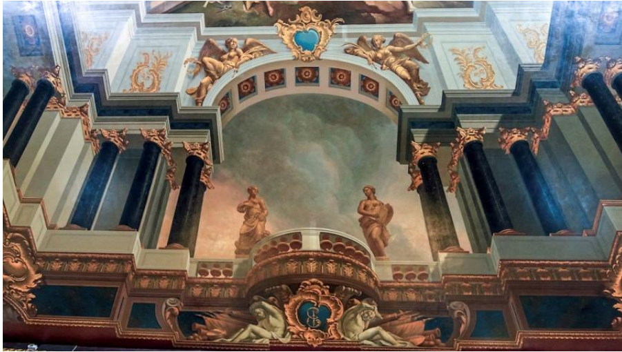
Figure 21. A fragment of the architectural detail of the Great Hall ceiling in colour
